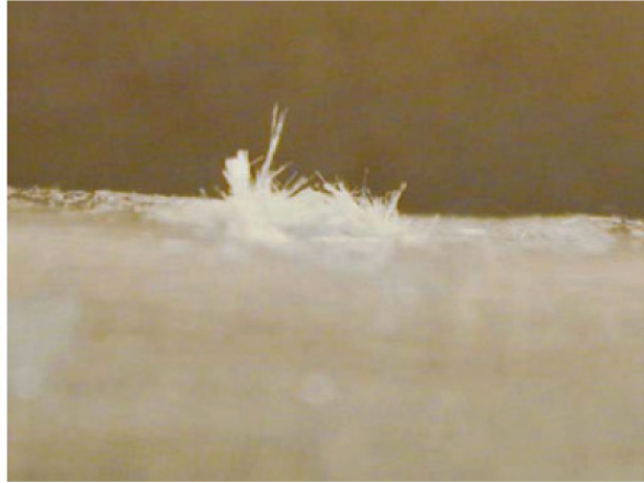
Figure C-3. Level 2 Damage/Defects: Penetration of Gel Coat (photo 3 of 3) Side view of damaged area showing some fiber breakage.
